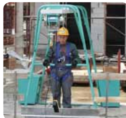
Gantry for stand hoists
